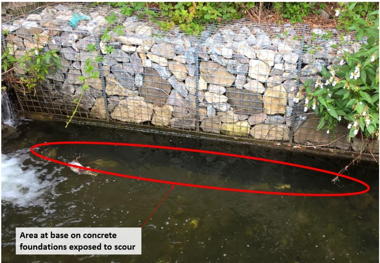
Figure 4 – Section 2: Gabion foundations exposed to scour
